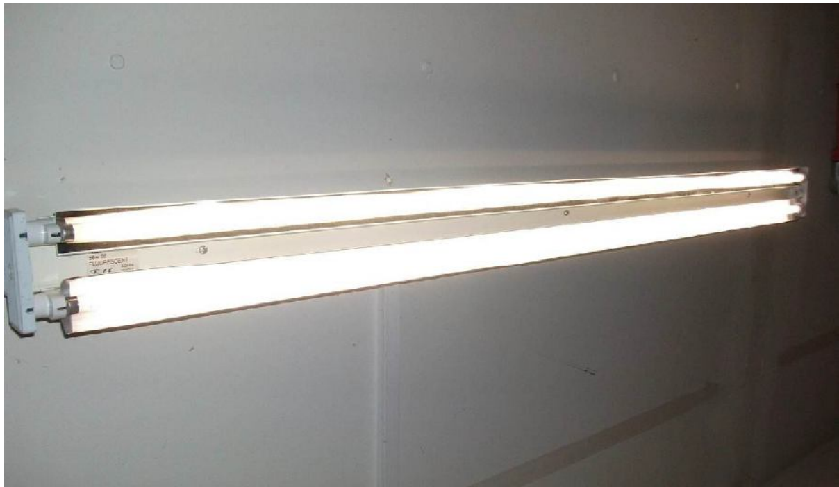
Figure 8 – Luminaire with T5 adapters and lamps
