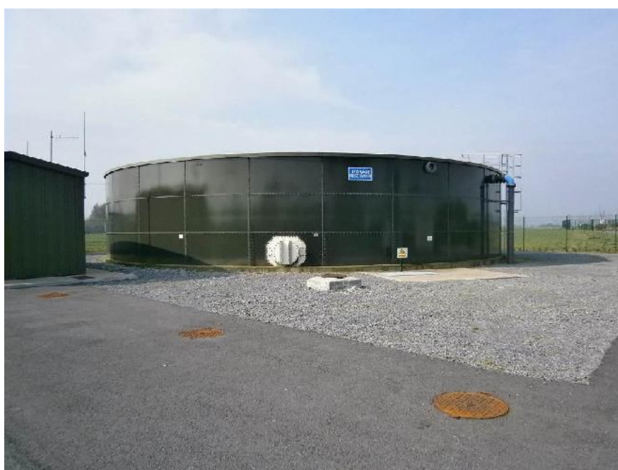
Figure 44 – Oak Park Water Treatment Plant Storage Reservoir
