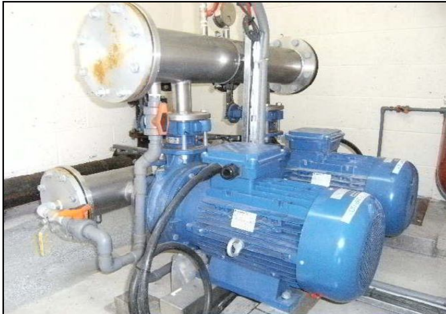
Figure 28 – Old 2 x 18.5kW Pumps - Royal Oak WTP
