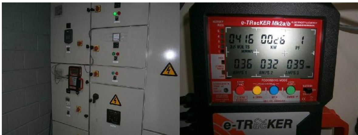
Figure 42 – E-tracker monitoring High Lift Pump 1
