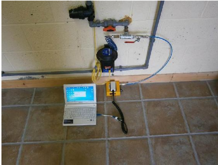
Figure 30 – Logging equipment Royal Oak WTP
