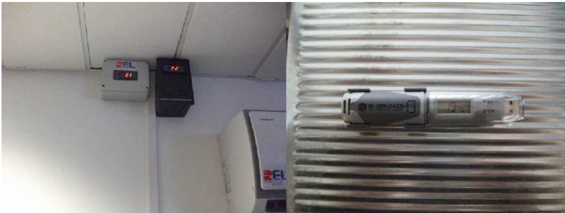
Figure 4 – Temperature / humidity sensors
