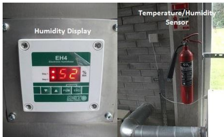
Figure 36 – Humidity Display and Sensor
