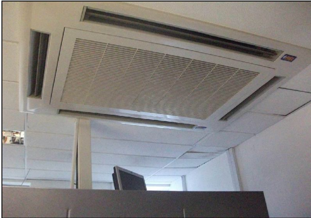
Figure 1 – Old 13kW fan coil air-conditioning unit
