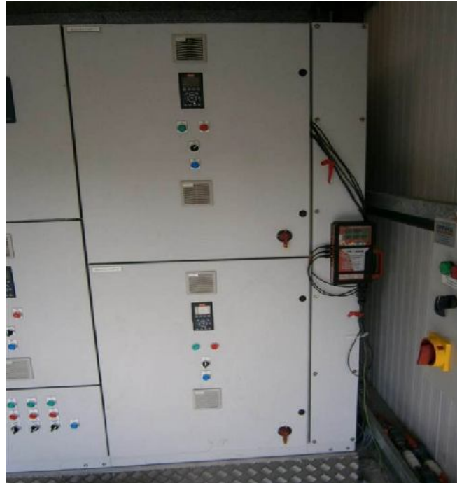
Figure 45 – Booster Pump 1 & 2 Control Panel
