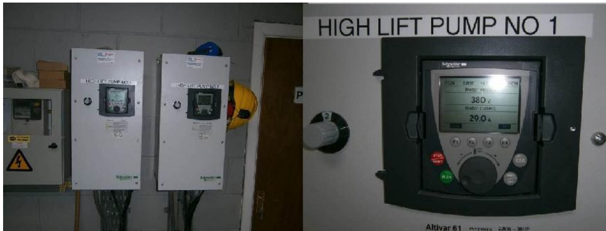
Figure 41 – VSDs for High Lift Pumps 1 & 2
