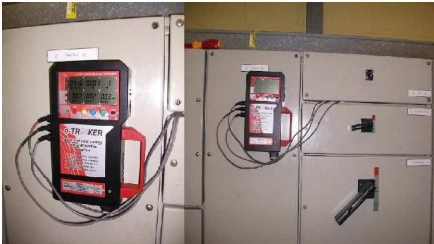
Figure 37 – e-Tracker monitoring power consumption of dehumidifier
