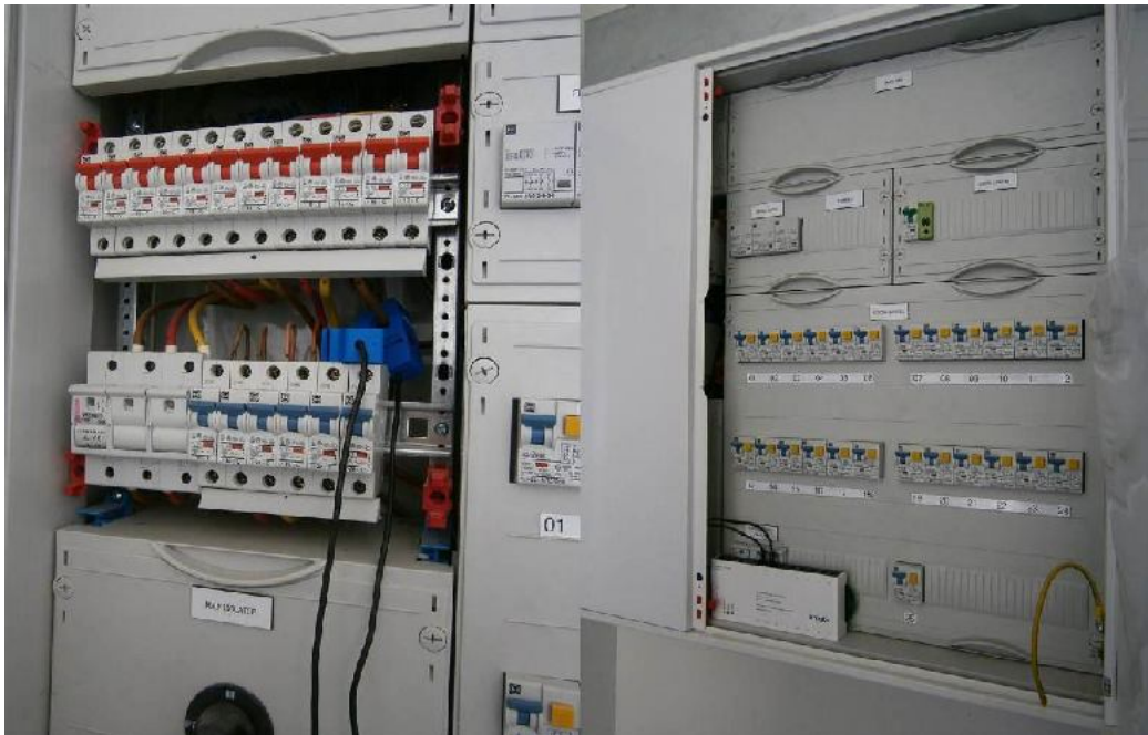
Figure 10 – Lighting Distribution Board with Enistic CT clamps
