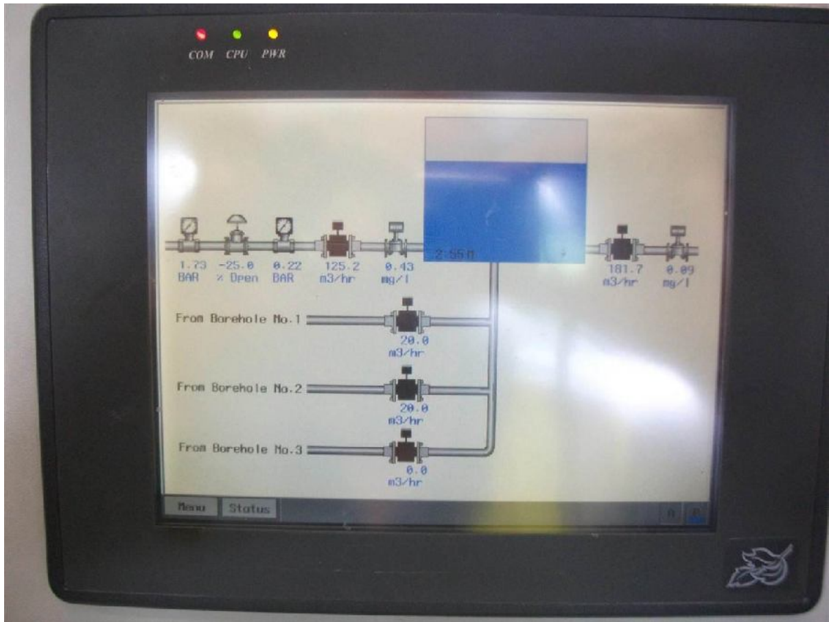
Figure 46 - HMI Oak Park Reservoir
