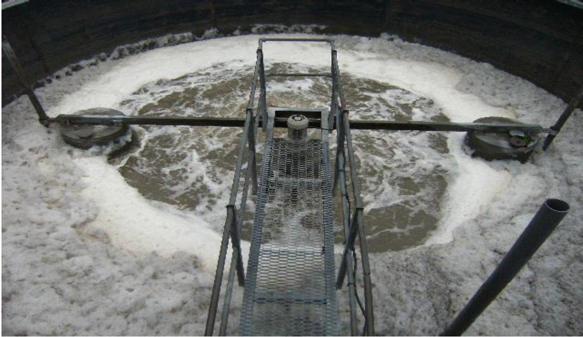
Figure 18 – Surface Aeration Venturi at Old Leighlin WWTP
