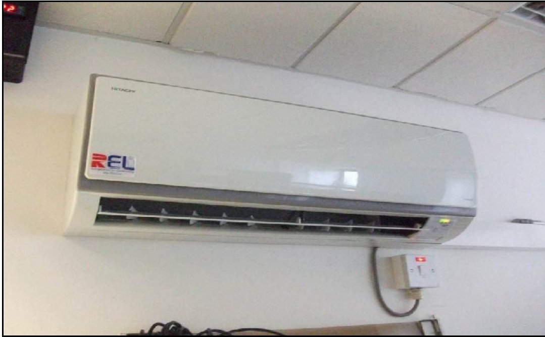
Figure 2 – New 6kW air-conditioning unit
