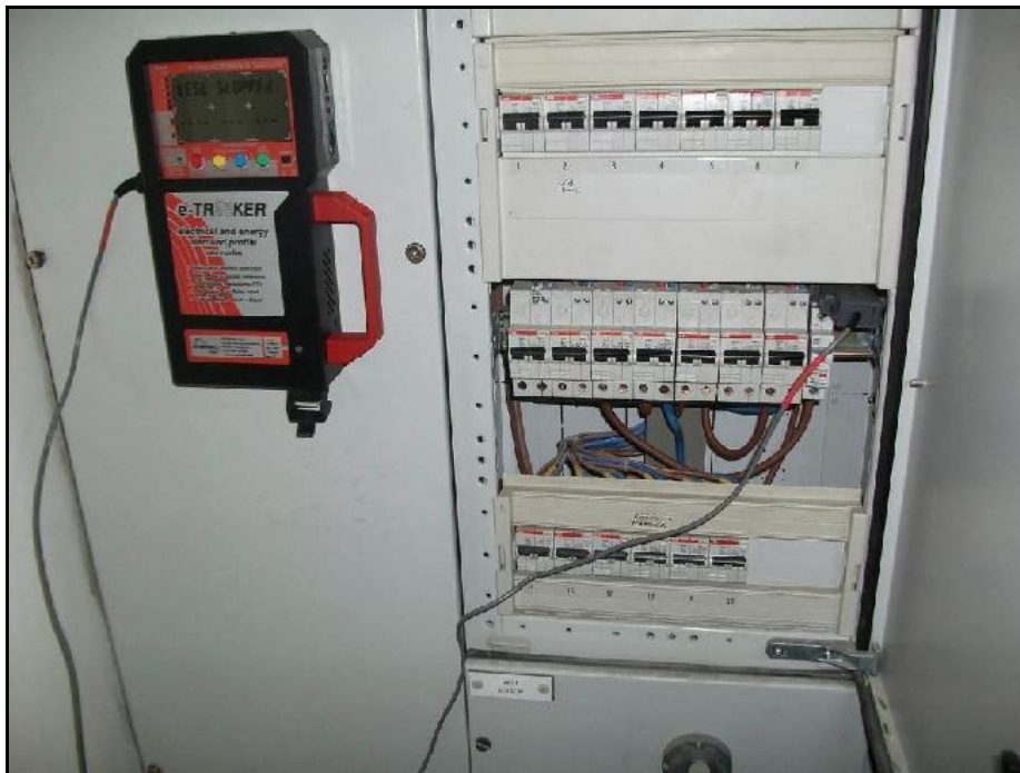
Figure 3 – E-tracker monitoring the air conditioning load
