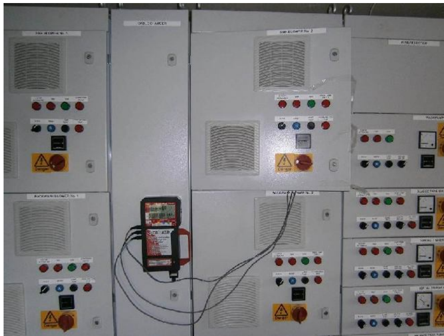
Figure 23 – Energy Monitoring at Rathoe WWTP
