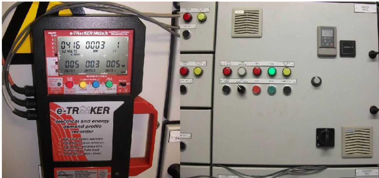
Figure 22 – Energy monitoring at Fenagh WWTP
